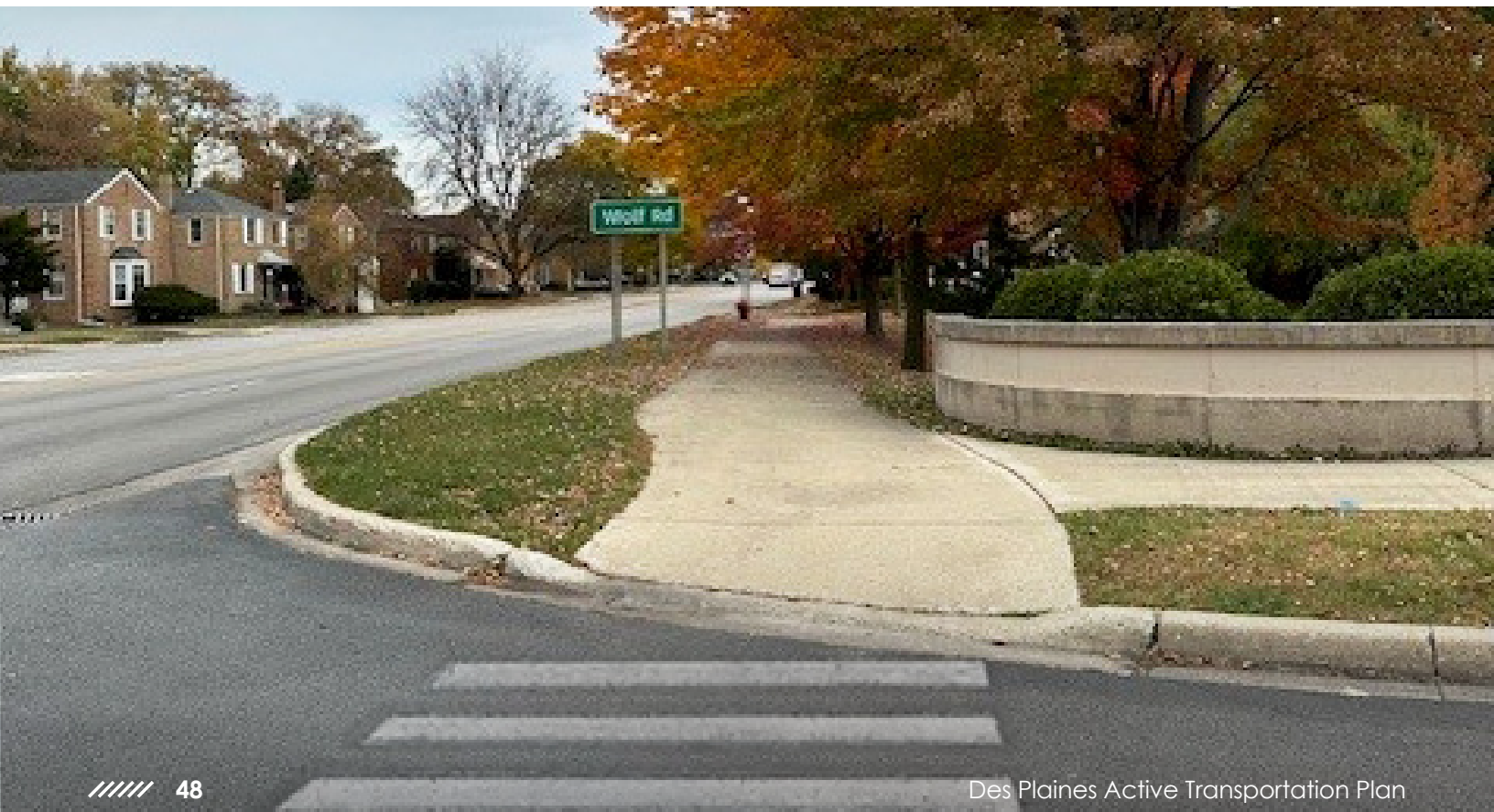
Shared use path on Thacker Street at the entrance to Prairie Lakes Park
